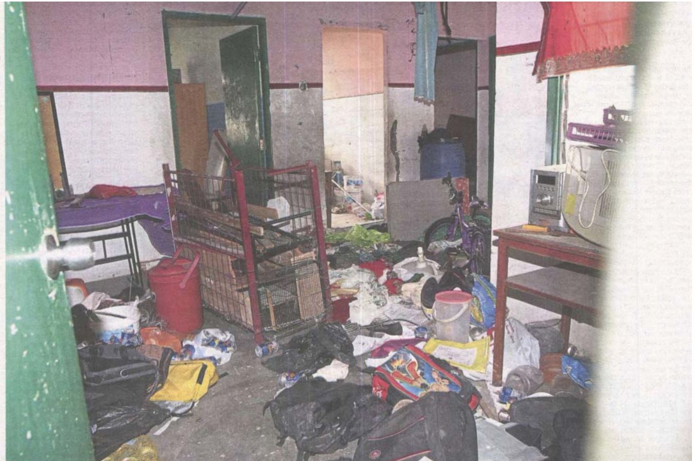
Rubbish haul: One of the abandoned apartment units in Palma Apartments in Bandar Country Homes, Rawang, that is used to store salvaged trash. This irresponsible act has resulted in insect infestation and rodents at the apartments. — Photo: AZLINA ABDULLAH/The Star
